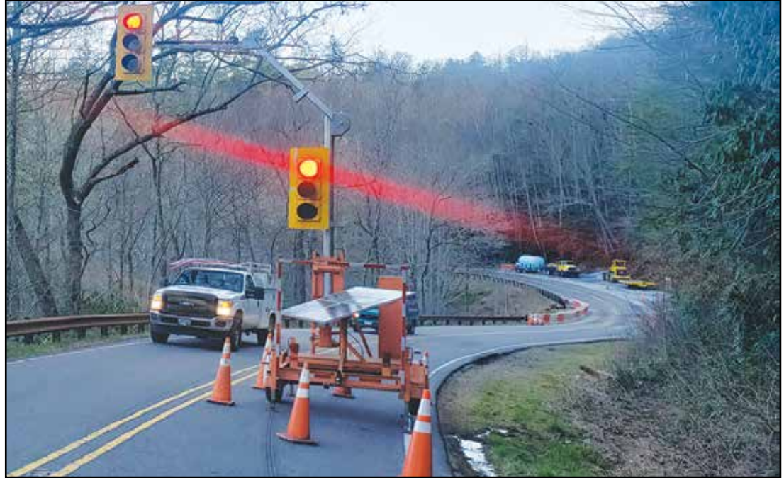
For a little over a week, motorist travelling US 64 west were greeted with traffic lights and one lane for travel but with work finishing up early, US 64 west is open and it's business as usual. – Photo by Kim Lewicki
