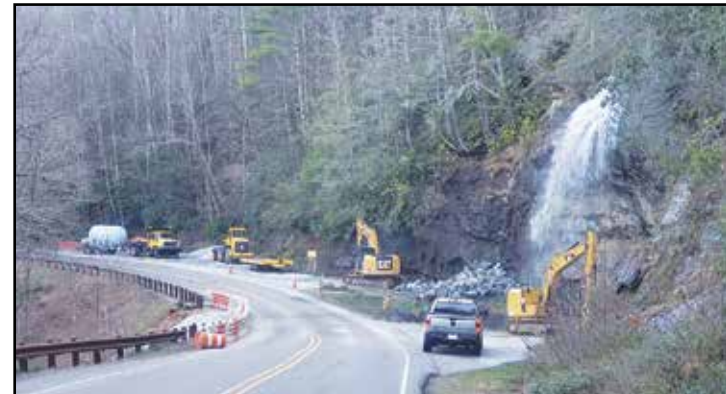
The drainage pipe under US 64 that carries water away from the falls was replaced and the embankment repaired – photo by Kim Lewicki
