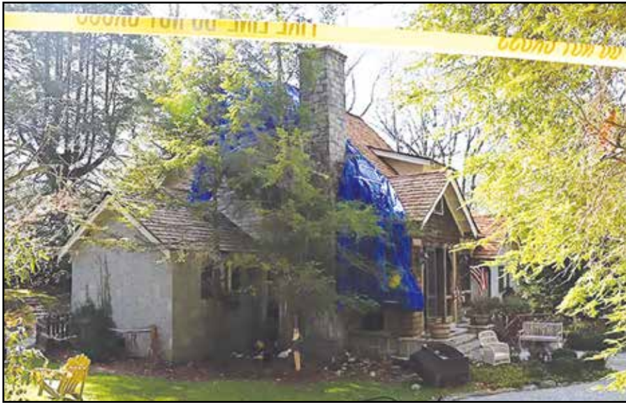
the home that caught fire on Nov. 21 and had minimal damage around the chimney.
