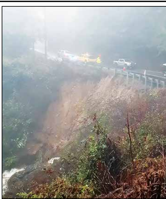
NC 106 (Dillard Road), Near Blue Valley Falls washed out 11 a.m., Thursday, Sept. 26 during the precursor front event before Hurricane Helene officially hit Highlands, early AM Friday, Sept. 27. According to NC DOT one lane near the washout is open with a temporary traffic light. Two lanes are open prior to and after the washout.
