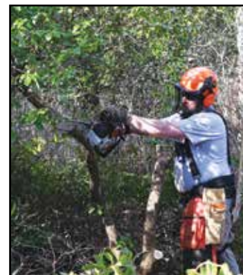
Creating a fire break included clearing dead trees and brush but also making room for rescue vehicles to maneuver in the area.
